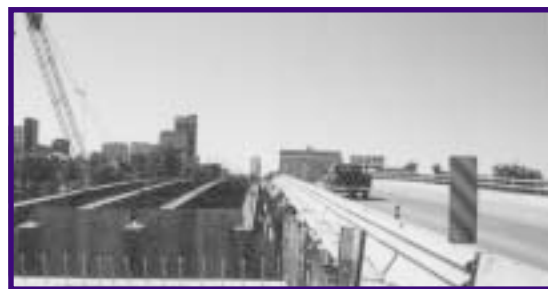
Dodge Street Bridge over I-480 in Omaha, Nebraska: Staged Construction in Progress.
